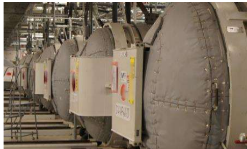
DUF6 plant is built to convert 46,000 cylinders of depleted uranium into more stable material
